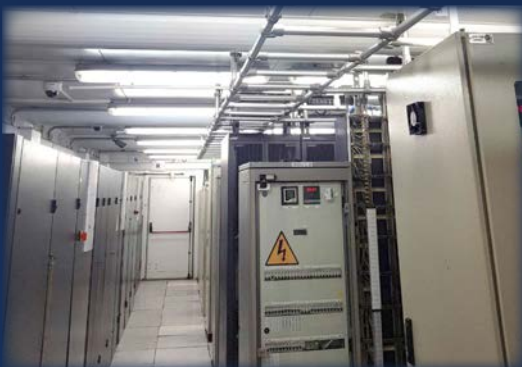
Project: Telecommunication containers laddering Location: Tabriz, Shiraz, Ahvaz, Karaj, Tehran, Babol, Esfahan, Mashhad Operator: MTNI
